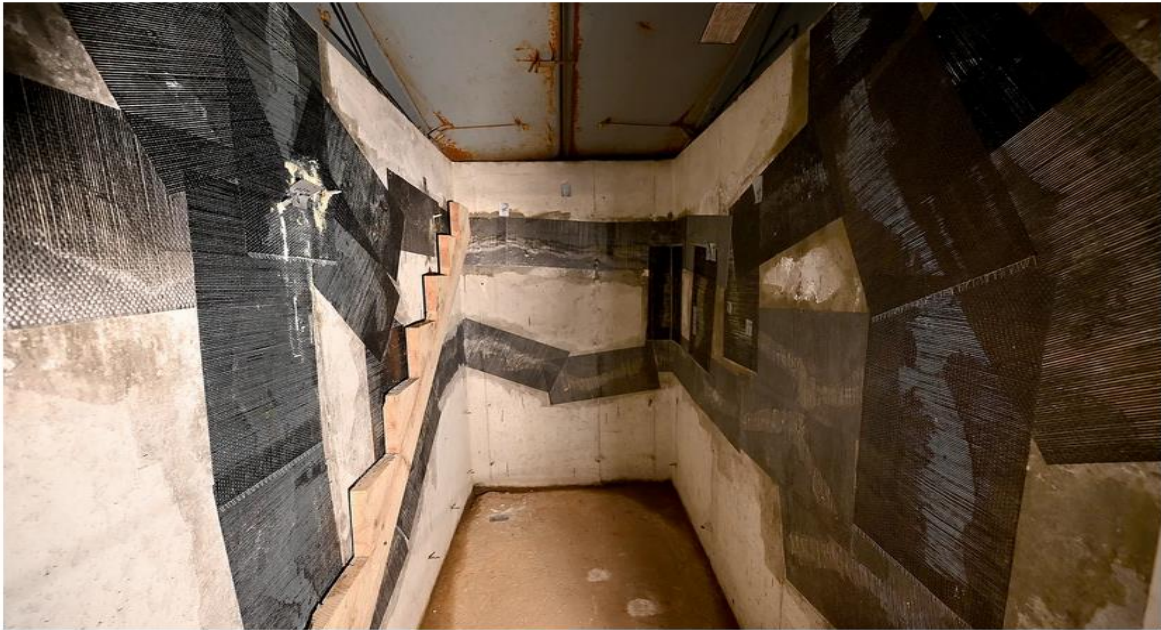
Gary Bellows uses carbon fiber to repair foundation cracks in the basement of his Rutland home. Cases of pyrrhotite-contaminated concrete foundations affect mainly Connecticut and Central Mass. towns, forcing homeowners to pay hundreds of thousands of dollars to repair or replace their foundations. Allan Jung/Telegram & Gazette, File
