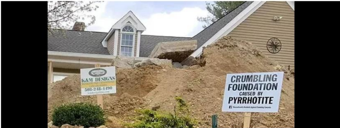
Cases of pyrrhotite-contaminated concrete foundations dot Connecticut and Central Mass. towns, including in Grafton, forcing homeowners to pay hundreds of thousands of dollars to repair or replace their foundations. T&G File Photo
