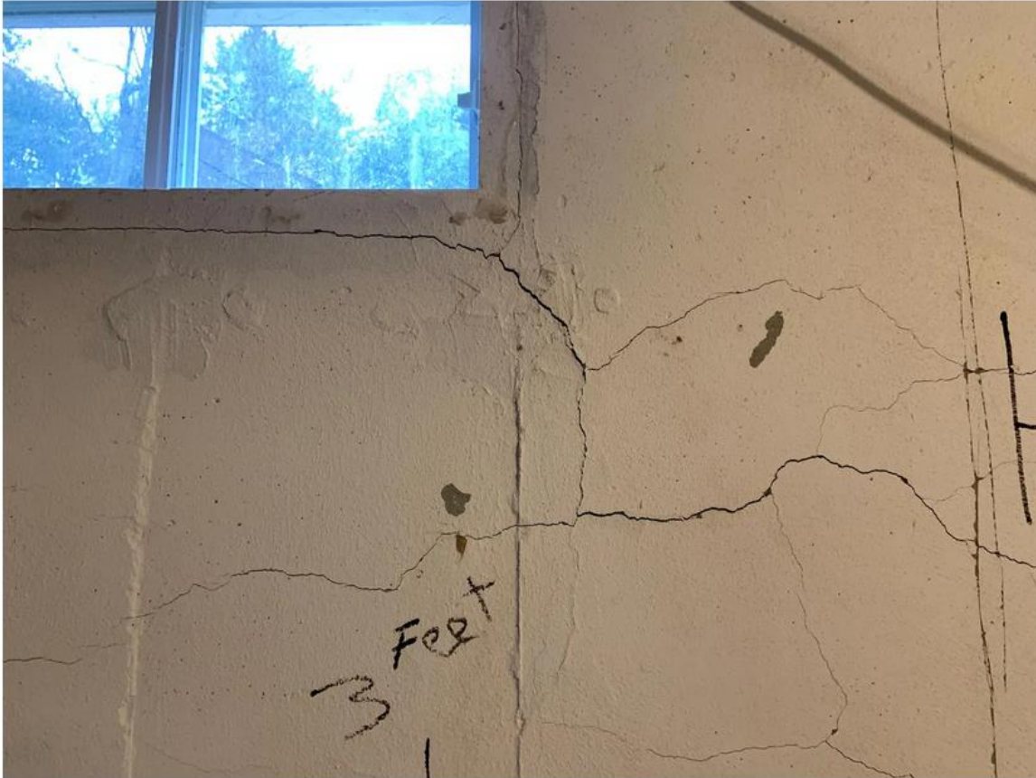
Telltale cracks in the foundation of a home in Holden. T&G File Photo
